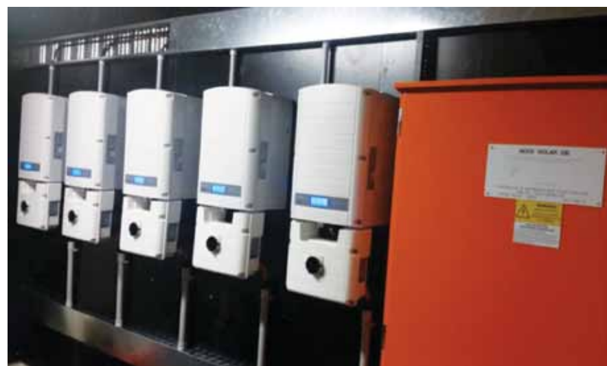
3-PHASE SOLAREEDGE INVERTERS AND AEES GROUP SOLAR DISTRIBUTION BOARD ALLOWING FOR SEAMLESS INTEGRATION OF THE SOLAR GENERATED-ELECTRICITY INTO THE CLUBHOUSE ELECTRICAL NETWORK, WITH ANY EXCESS GENERATED-ELECTRICITY SENT TO THE GRID
